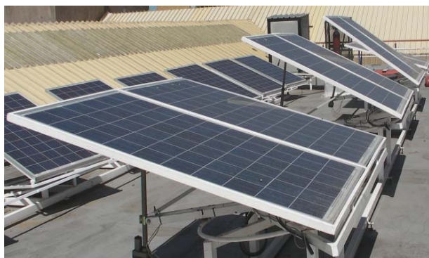
Figure 15. Three identical solar panels set to tilt angles of 16°, 26° and 36° degrees.
