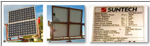
Figure 19. The solar panels.
