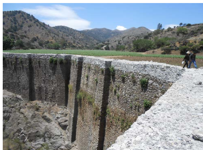
Figure 8. El Saucillo dam, augmentation of a spillway water curtain (Galindo 2015).
