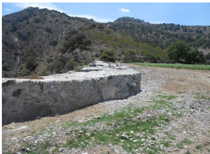
Figure 7. El Saucillo dam, augmentation of a spillway water curtain (Galindo 2015).
