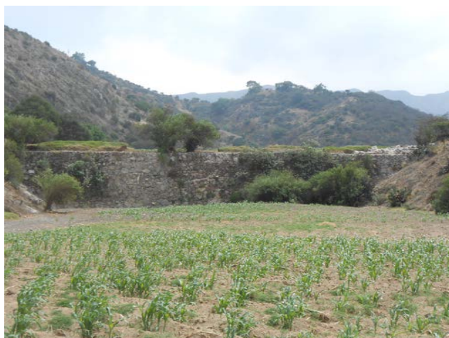
Figure 4. Front view of a wall in the interior of a dam (Galindo 2015).
