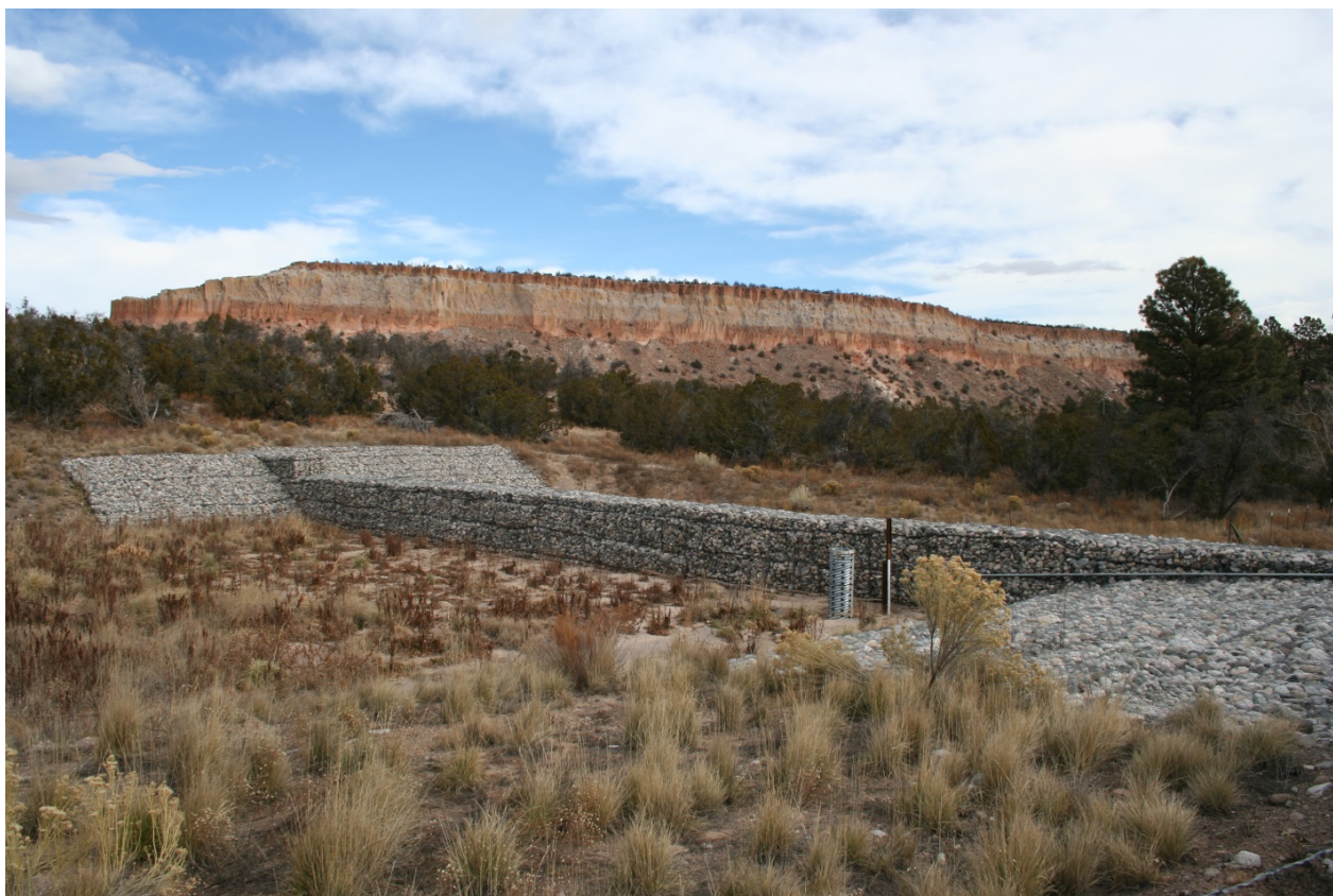
Figure 2. The Los Alamos Canyon sediment retention structure (upgradient side) in 2005 near the northeastern boundary of Los Alamos National Laboratory.
