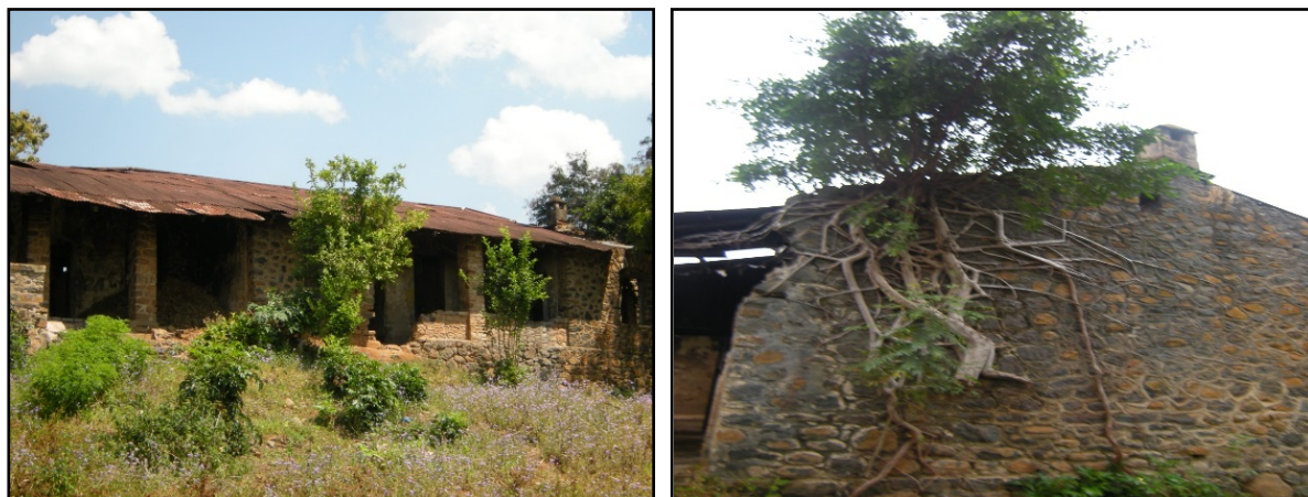
Plate 4. Deterioration conditions: trees are cropping up on the walls of the historic German Boma in Masoko.
