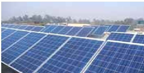
15 KW-Mobile Communications India Limited, New Delhi [15], Coursty: Radiant solar.
