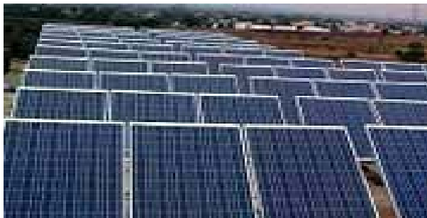
25 KW-Sagar Group of Institution, Hyderabad [15], Coursty: Radiant solar.
