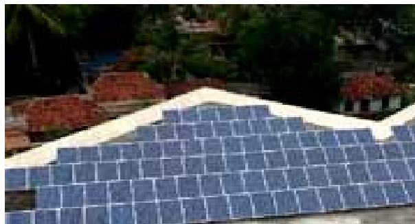
100 KW-Pushpagiri Institute of Medical Science and Research Centre, Tiruvalla Coursty: Radiant solar [15].
