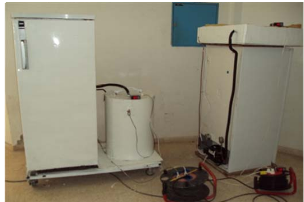
Figure 15. Photographs of the two refrigerators: One coupled with the water-heater, the other with the heating floor.
